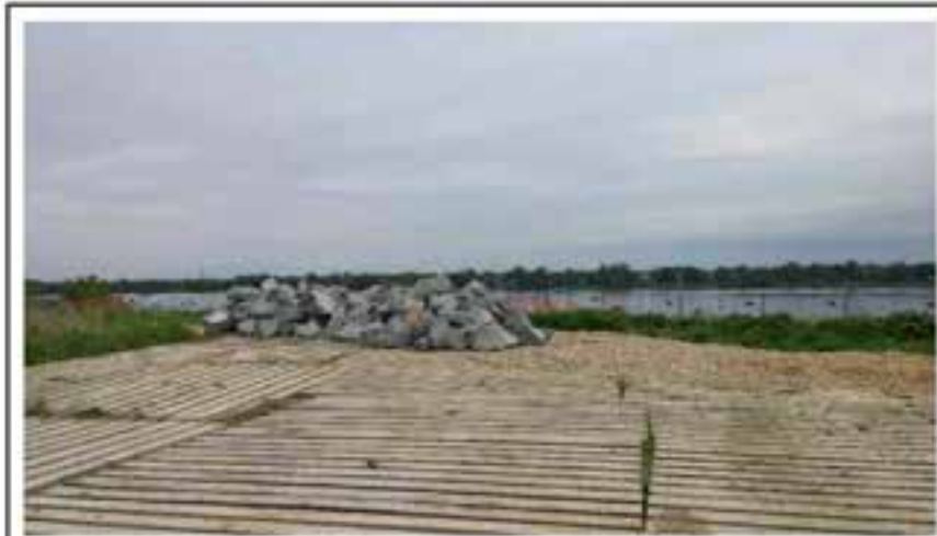
Photo 3: R6 material stockpile on top of crushed stone pad at end of site access road, facing northeast.
