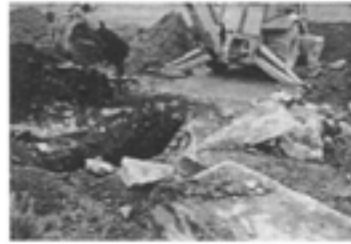
Figure 5. Uncovering the UST during the 1999 Pre -Design Investigation, note the oily (dark) quality of the subsurface soil
